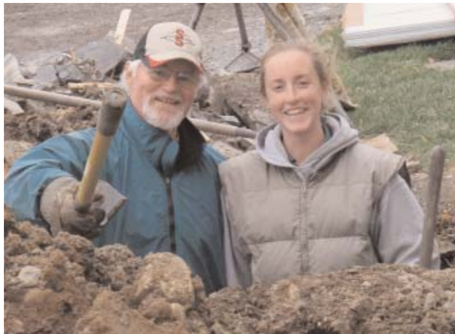
Newly-minted farmstead cheese owner Keeley McGarr gets her hands dirty during the renovation process with help from her father, Dan McGarr, former president of the New York Holstein Association and an international dairy show judge. Keeley Cheese Co. opens this month, bringing washed rind artisan cheese to New York state's Finger Lakes region.
